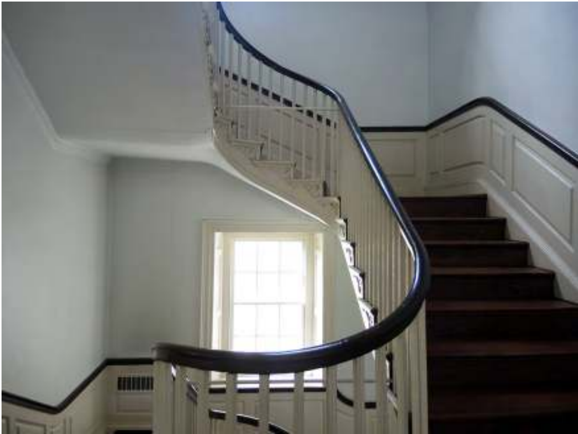
PHOTO 154 - Main Block Interior, Room 202, Looking Southwest; Damage to Plaster Above Window and Wood Window Trim (09-13-2016, ...
