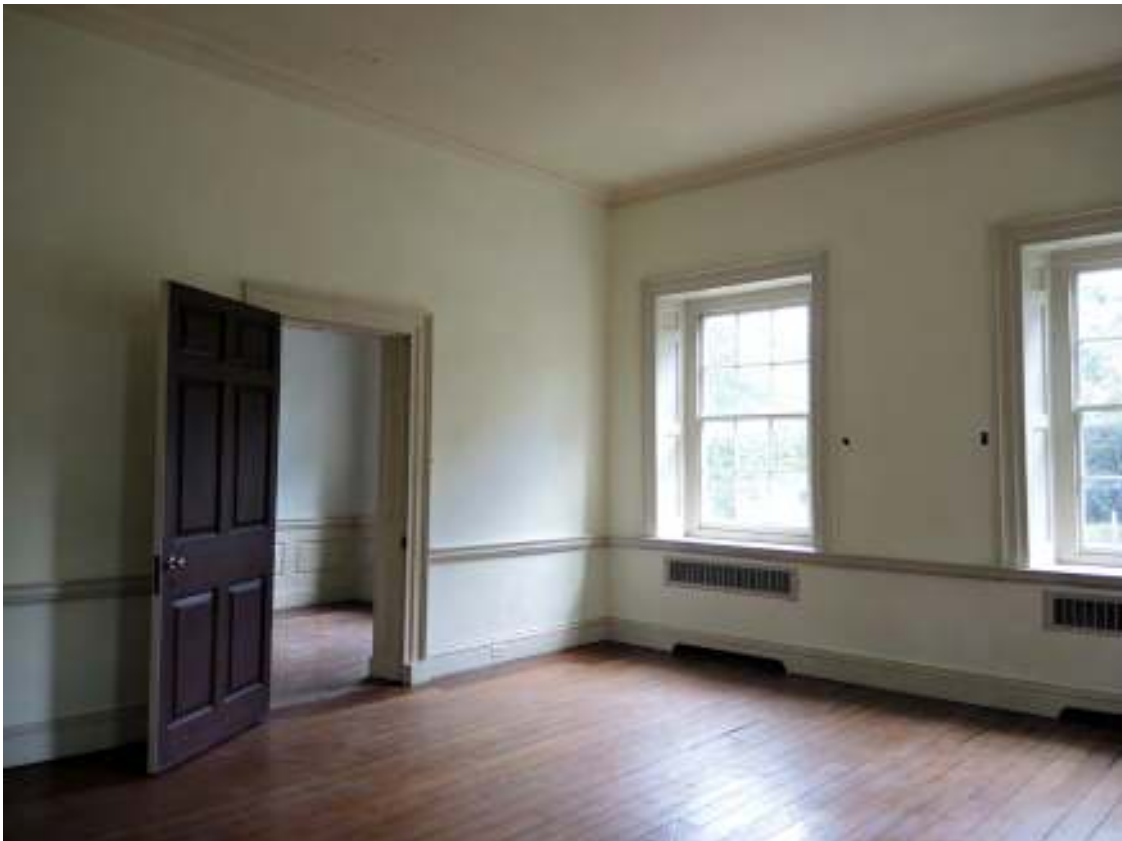
PHOTO 106 - Main Block Interior, Room 201, Northwest Corner; Plaster Molding Damage on West Wall (09-13-2016, NTHP)
