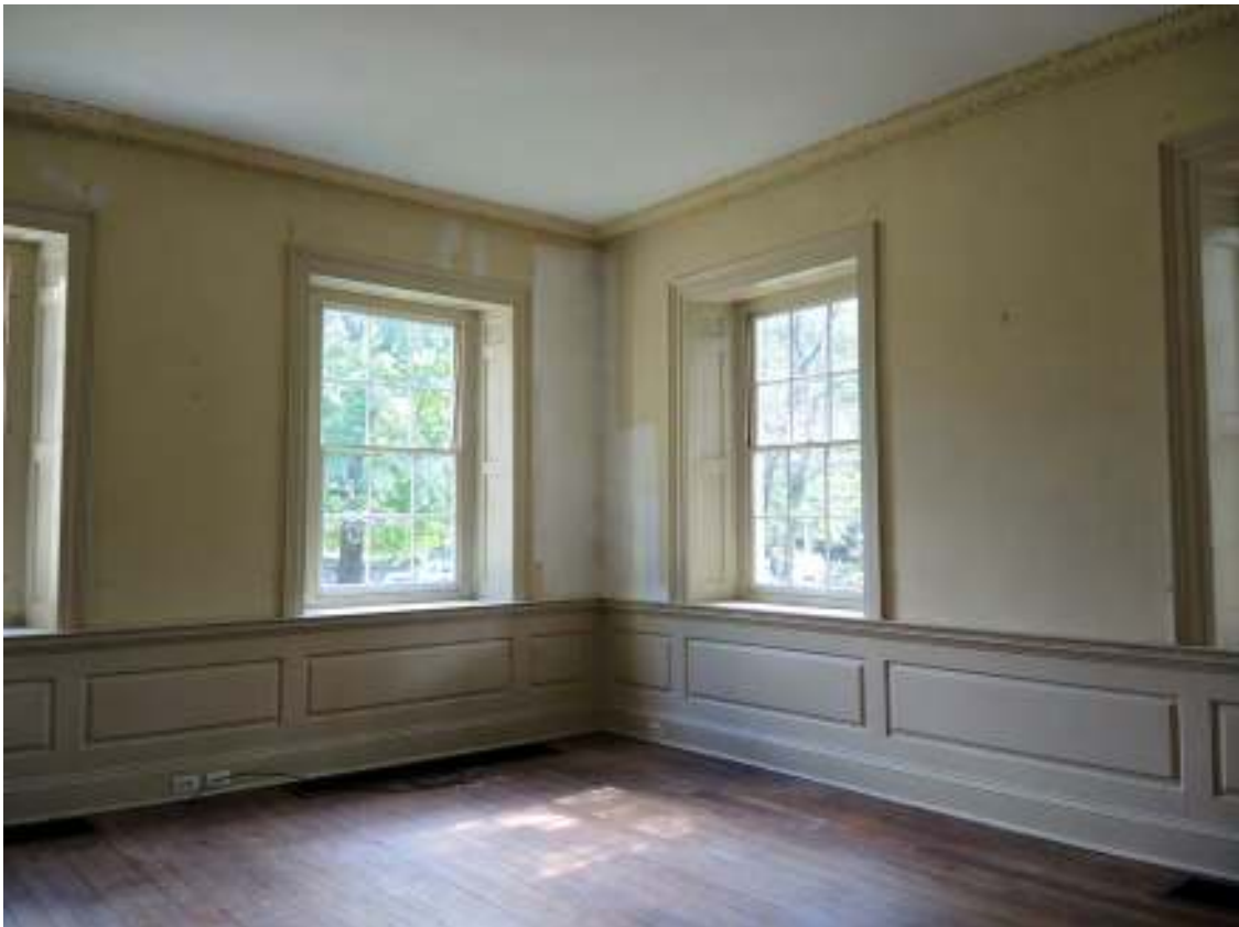
PHOTO 064 - Main Block Interior, Room 101, Northeast Corner; Plaster Damage on North Wall and Molding (09-13-2016, NTHP)
