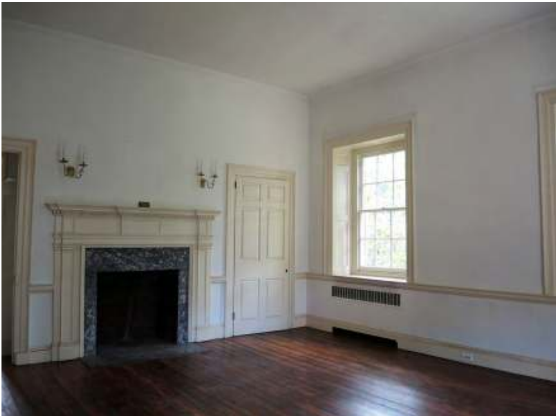
PHOTO 116 - Main Block Interior, Room 204, Northeast Corner; Cracks in Stone Fireplace Surround, Cracked Plaster on Walls and Molding...
