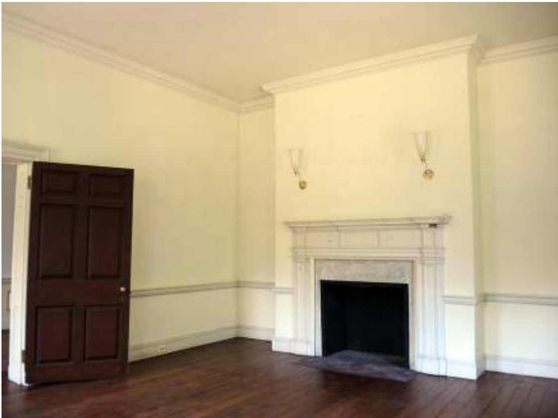
PHOTO 114 - Main Block Interior, Room 203, Southeast Corner; Cracked Plaster Molding and Ceiling on East Wall (09-13-2016, NTHP)
