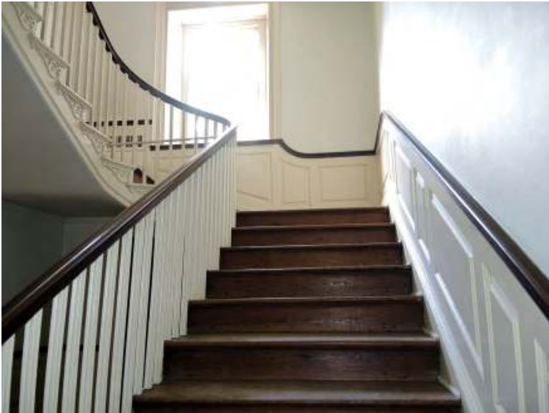
PHOTO 059 - Main Block Interior, Room 102, Looking Southwest; Hole in Floors at Northwest Corner of First Landing (09-13-2016, NTHP)
