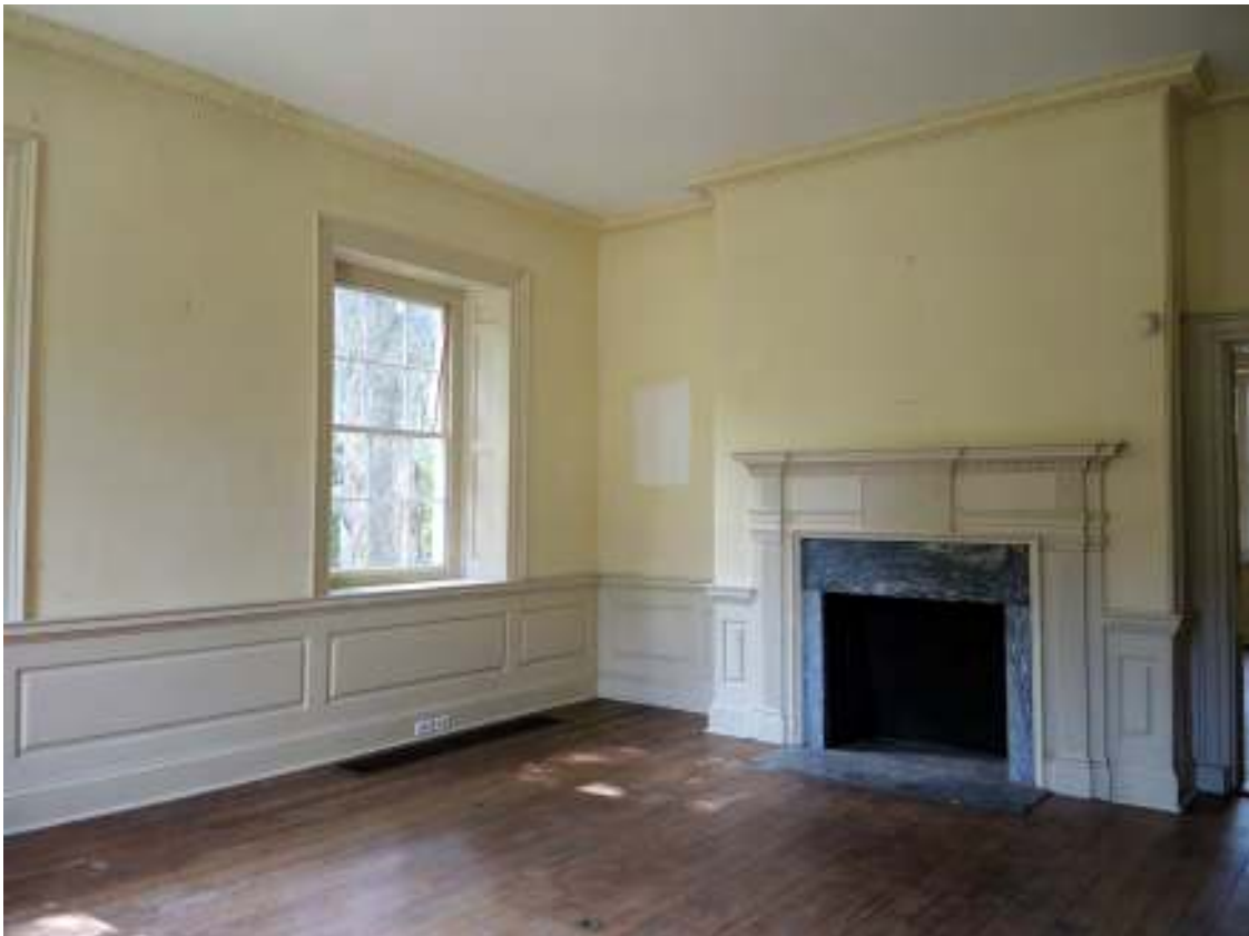
PHOTO 060 - Main Block Interior, Room 101, Southeast Corner; Gap in Top Rail & Wainscotting at Corner, Plaster Molding Damage at East...
