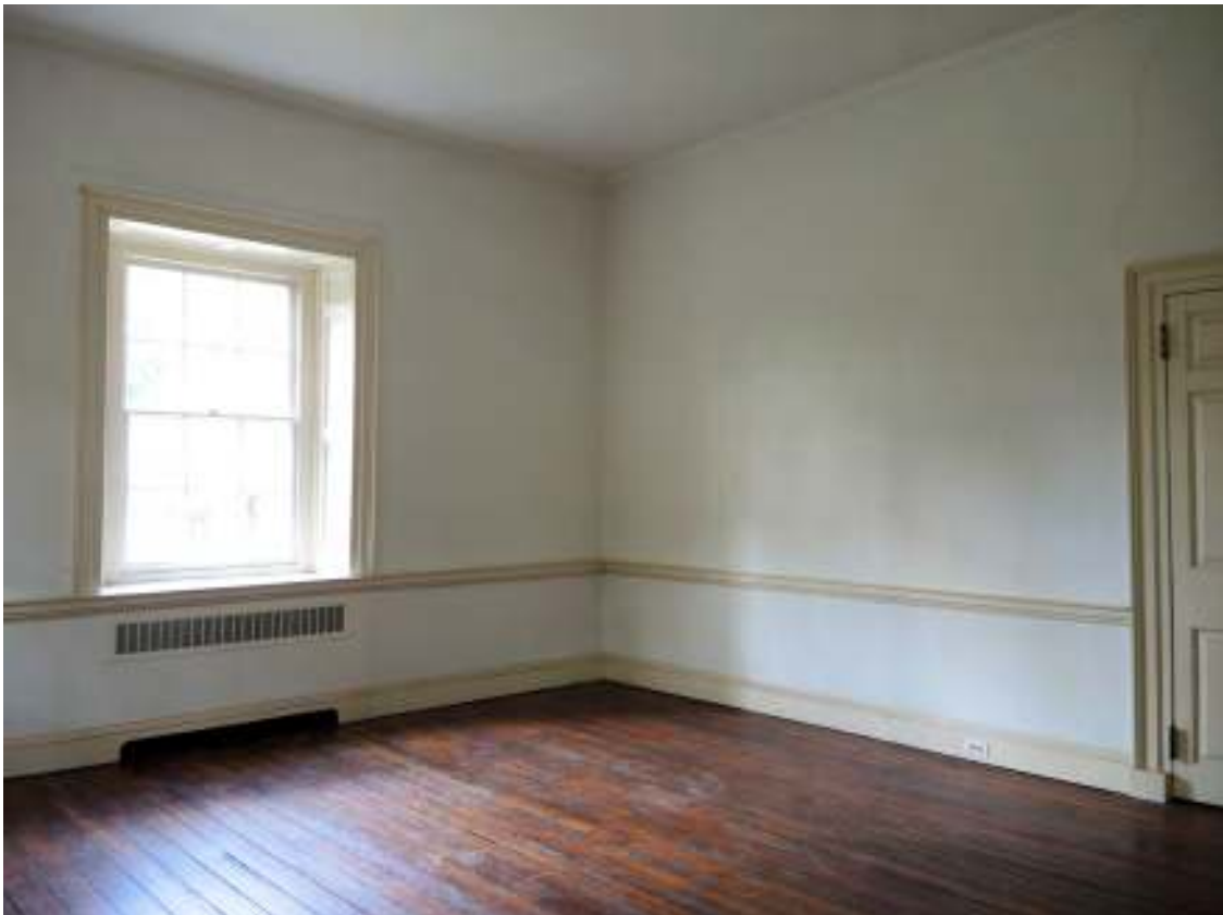
PHOTO 118 - Main Block Interior, Room 204, Southwest Corner; Cracked Plaster Along Ceiling at South Wall (09-13-2016, NTHP)
