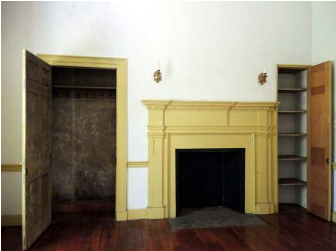
PHOTO 125 - Main Block Interior, Room 205, North Wall; Damaged Plaster above West Door, Fireplace Surround Split Wood, Peeling Paint...
