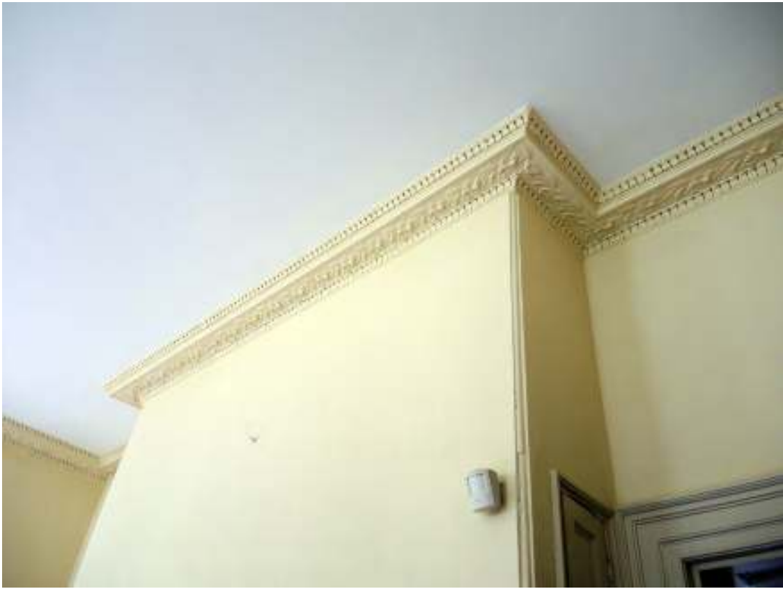
PHOTO 067 - Main Block Interior, Room 101, Detail of Plaster (09-13-2016, NTHP)
