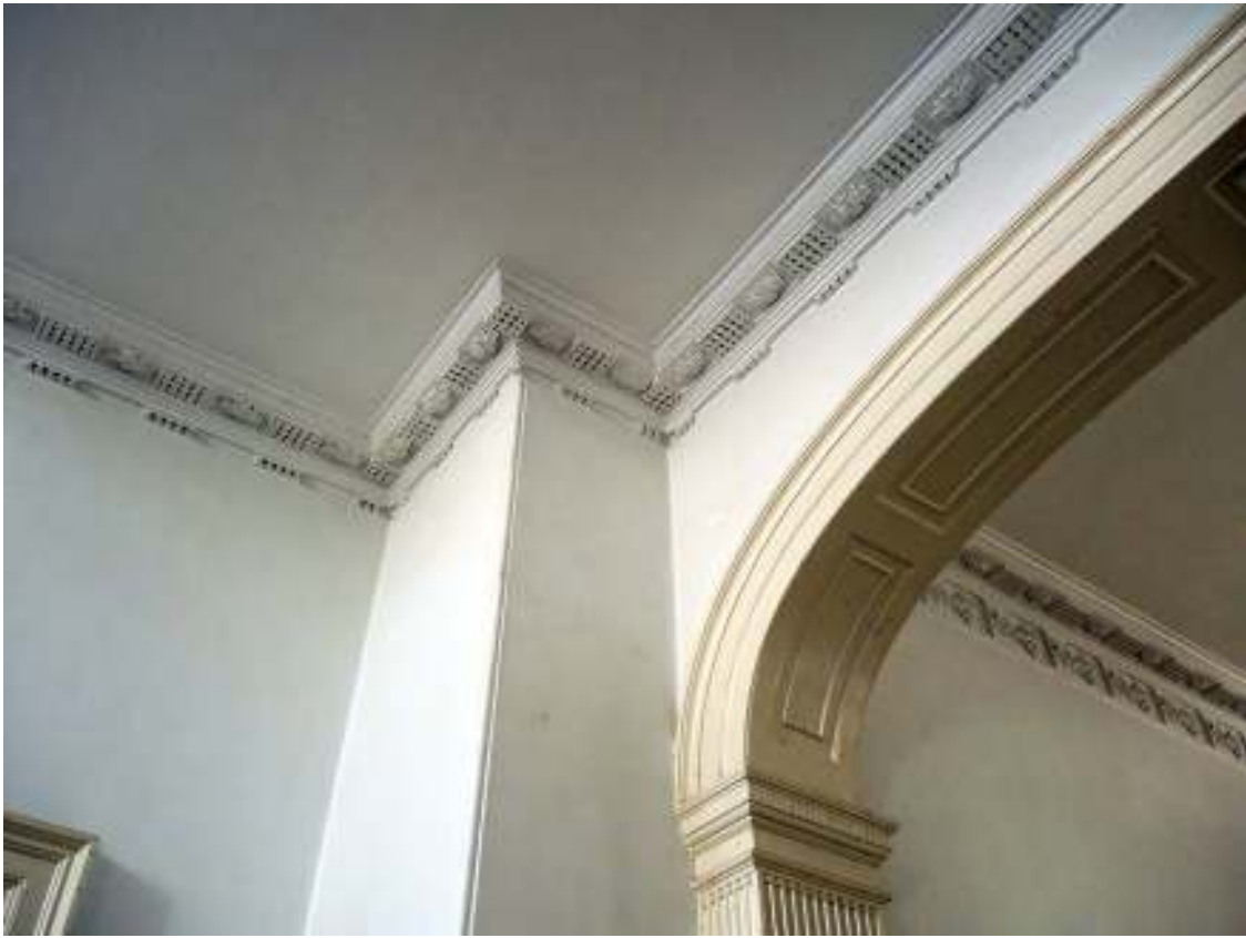
PHOTO 053 - Main Block Interior, Room 102, Detail of Plaster and Millwork; Crack in Northeast Corner of Wooden Arch (09-13-2016, NTHP)
