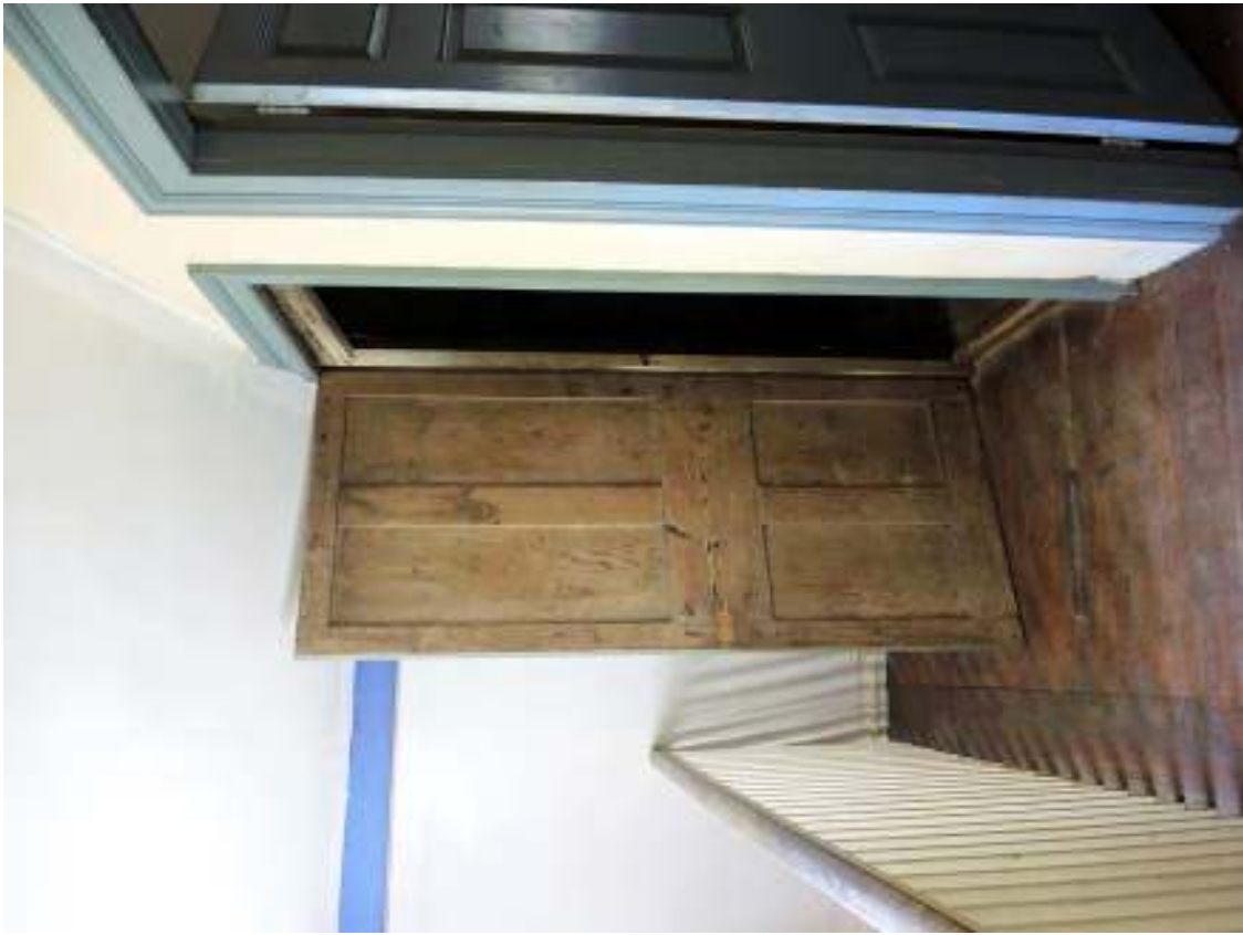
PHOTO 150 - Rear Extension Interior, Room 209A, Looking Southwest; Damaged Wood Floors (09-14-2016, NTHP)
