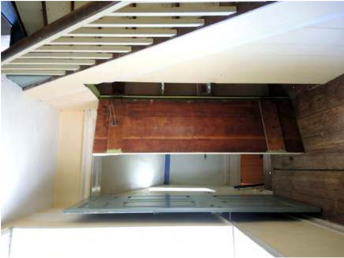
PHOTO 146 - Ell Interior, Room 209, Looking West; Hole in Center of Floor (09-14-2016, NTHP)
