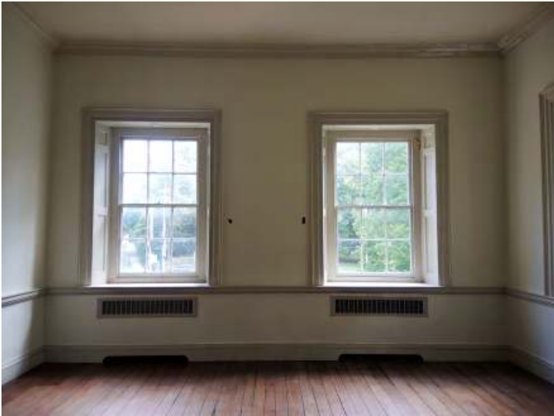
PHOTO 107 - Main Block Interior, Room 201, North Wall; Plaster Molding Damage at East Corner (09-13-2016, NTHP)
