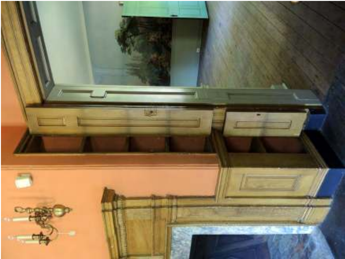
PHOTO 073 - Main Block Interior, Room 103, Detail of West Cabinet; Cabinet Hardware Missing (09-13-2016, NTHP)
