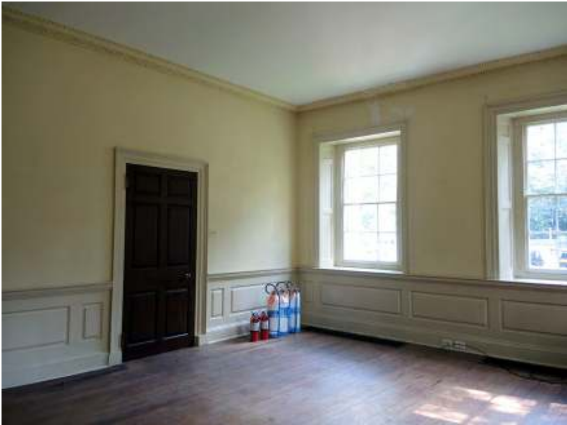
PHOTO 063 - Main Block Interior, Room 101, Northwest Corner; Plaster Molding Damage on North Wall (09-13-2016, NTHP)
