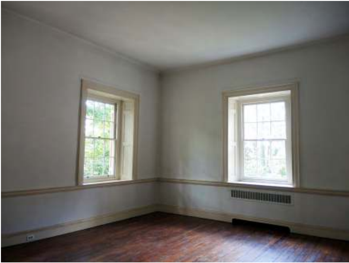
PHOTO 117 - Main Block Interior, Room 204, Southeast Corner; Cracked Plaster above South Window (09-13-2016, NTHP)
