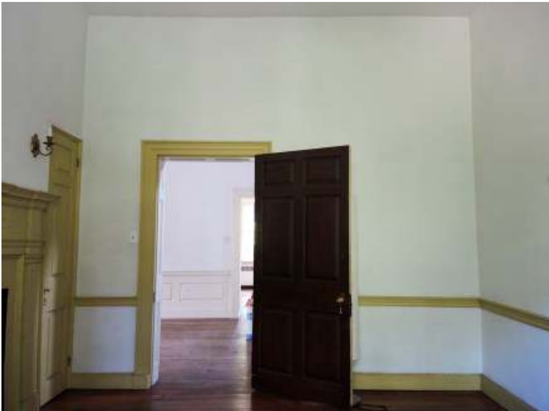
PHOTO 127 - Main Block Interior, Room 205, East Wall; Cracked Plaster at top of East Wall (09-13-2016, NTHP)
