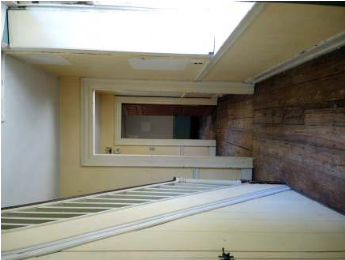
PHOTO 148 - Ell Interior, Room 209, Looking Northeast; Damaged Wood Floors (09-14-2016, NTHP)
