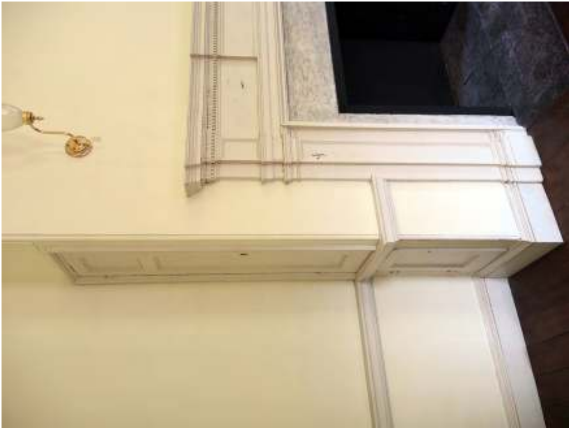
PHOTO 115 - Main Block Interior, Room 203, Detail of Cabinet; Flaking Paint on Wood Fireplace Mantel (09-13-2016, NTHP)
