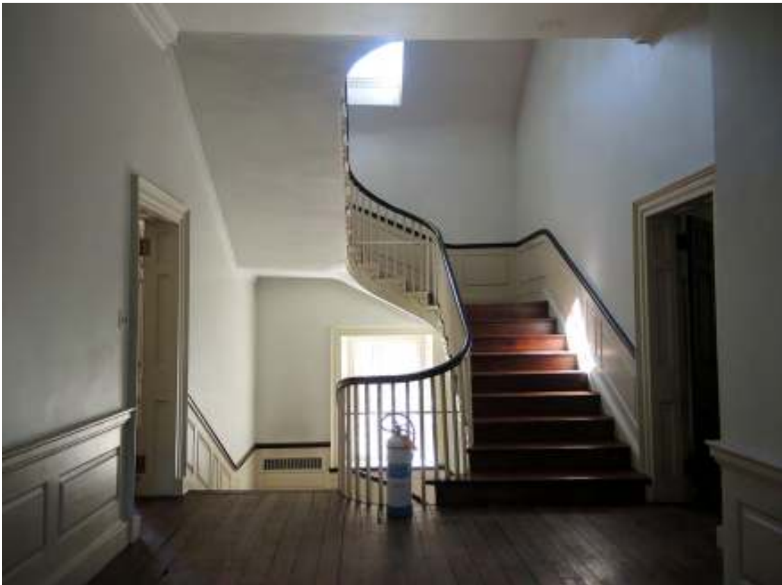
PHOTO 104 - Main Block Interior, Room 202, Looking Southwest; Cracks at Underside of Staircase Extending to East Wall above Door (09-...
