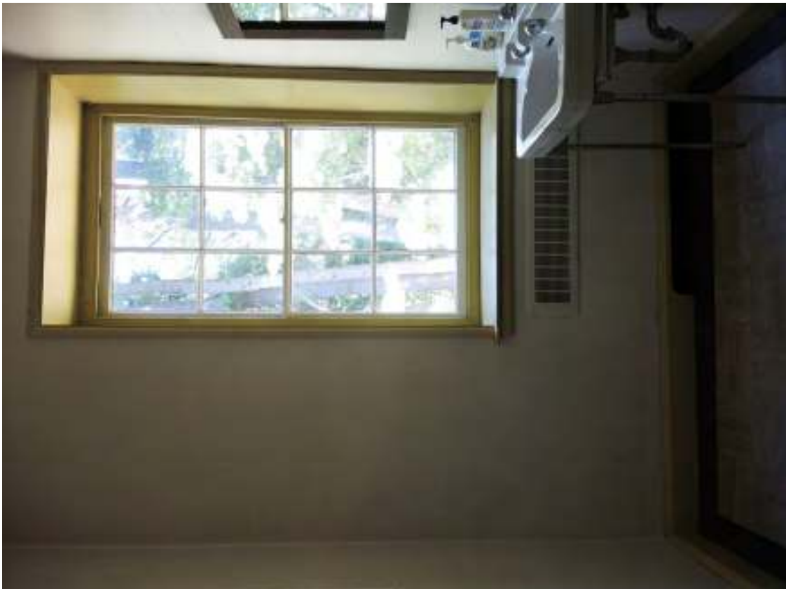
PHOTO 129 - Main Block Interior, Room 205A, West Wall; Ceiling Damage, Cracked Plaster Above Sink on North Wall (09-14-2016, NTHP)
