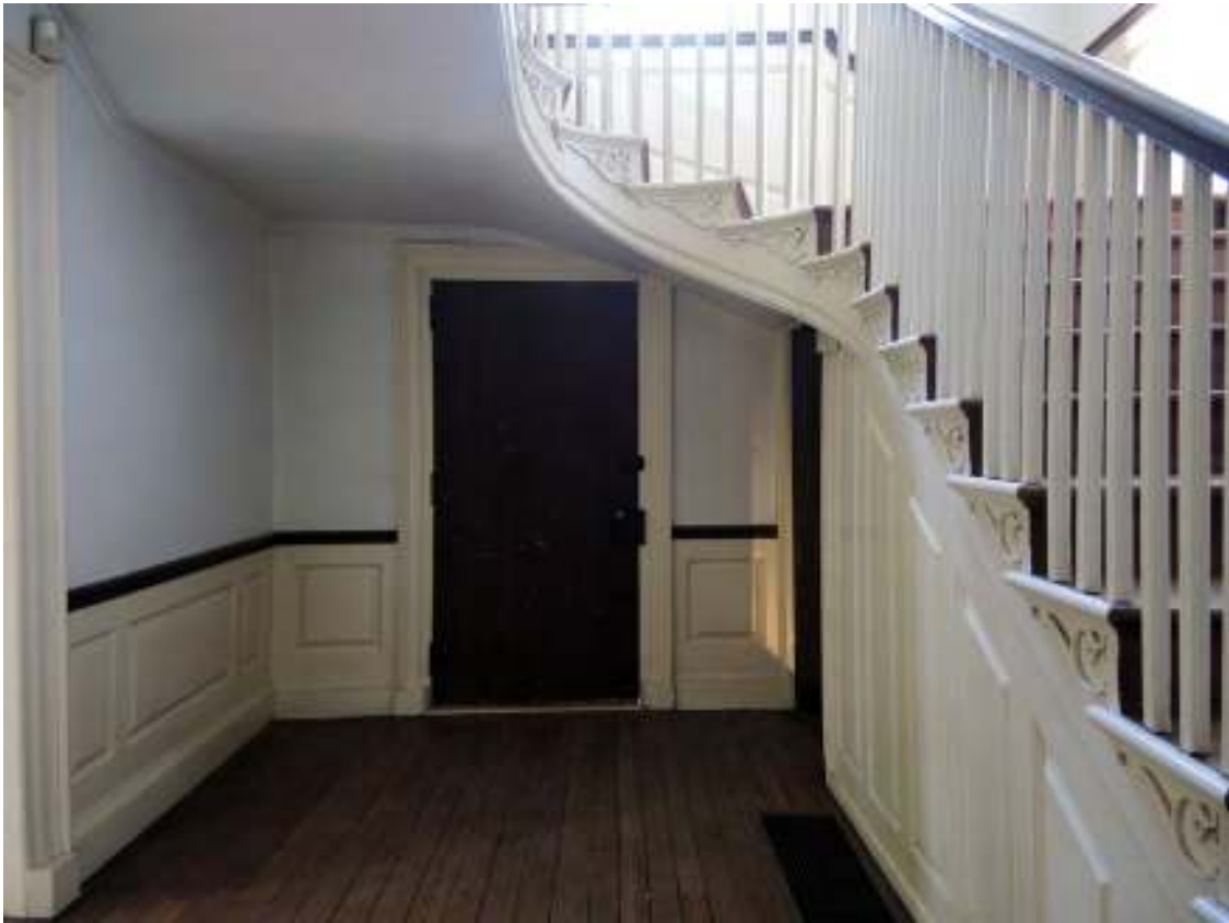
PHOTO 051 - Main Block Interior, Room 102, Looking Southwest; Cracked Plaster Underside of Staircase (09-13-2016, NTHP)
