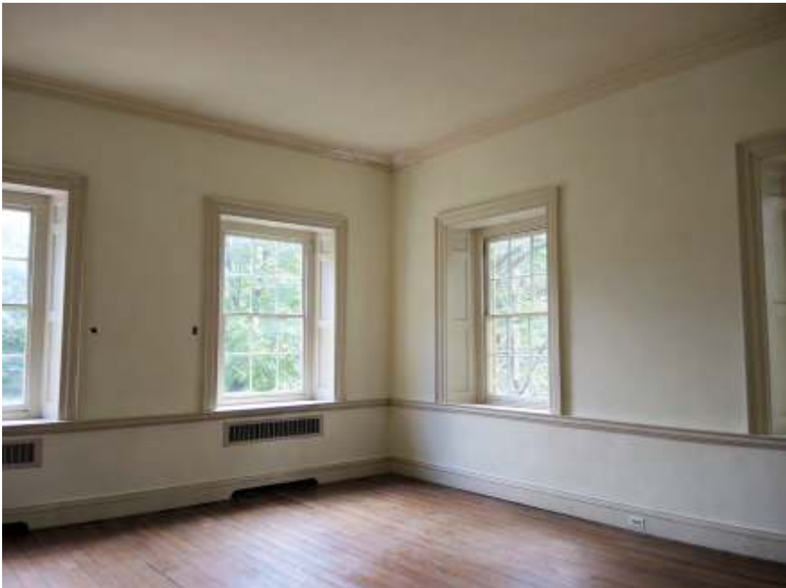
PHOTO 108 - Main Block Interior, Room 201, Northeast Corner; Plaster Molding Damage at Corner (09-13-2016, NTHP)
