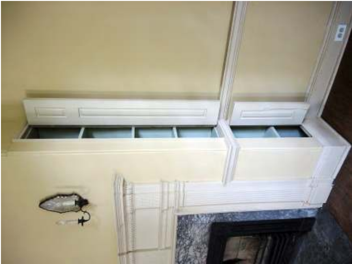
PHOTO 079 - Main Block Interior, Room 104, Detail of East Cabinet; Cracked Plaster Above Cabinet (09-13-2016, NTHP)
