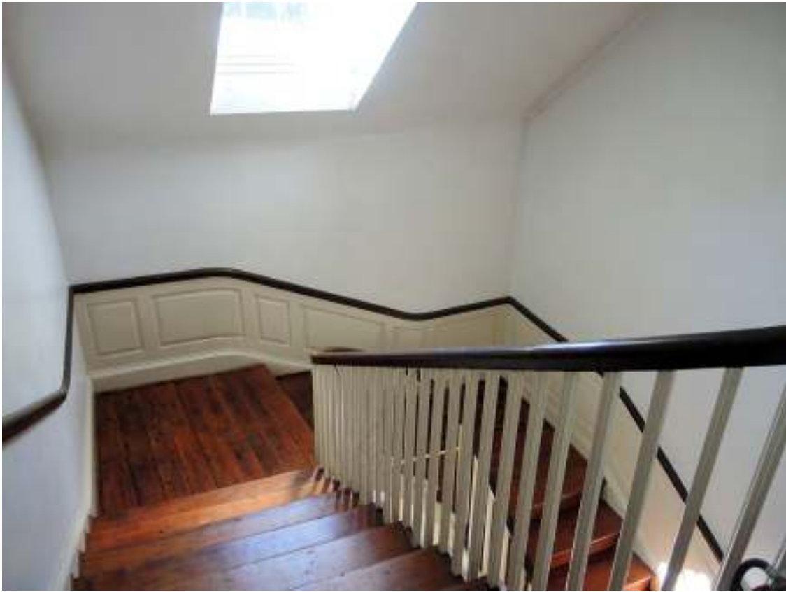
PHOTO 158 - Main Block Interior, Room 302, Looking Southwest; Cracked Plaster in West Corner, Plaster Damage at Dormer (09-14-2016,...
