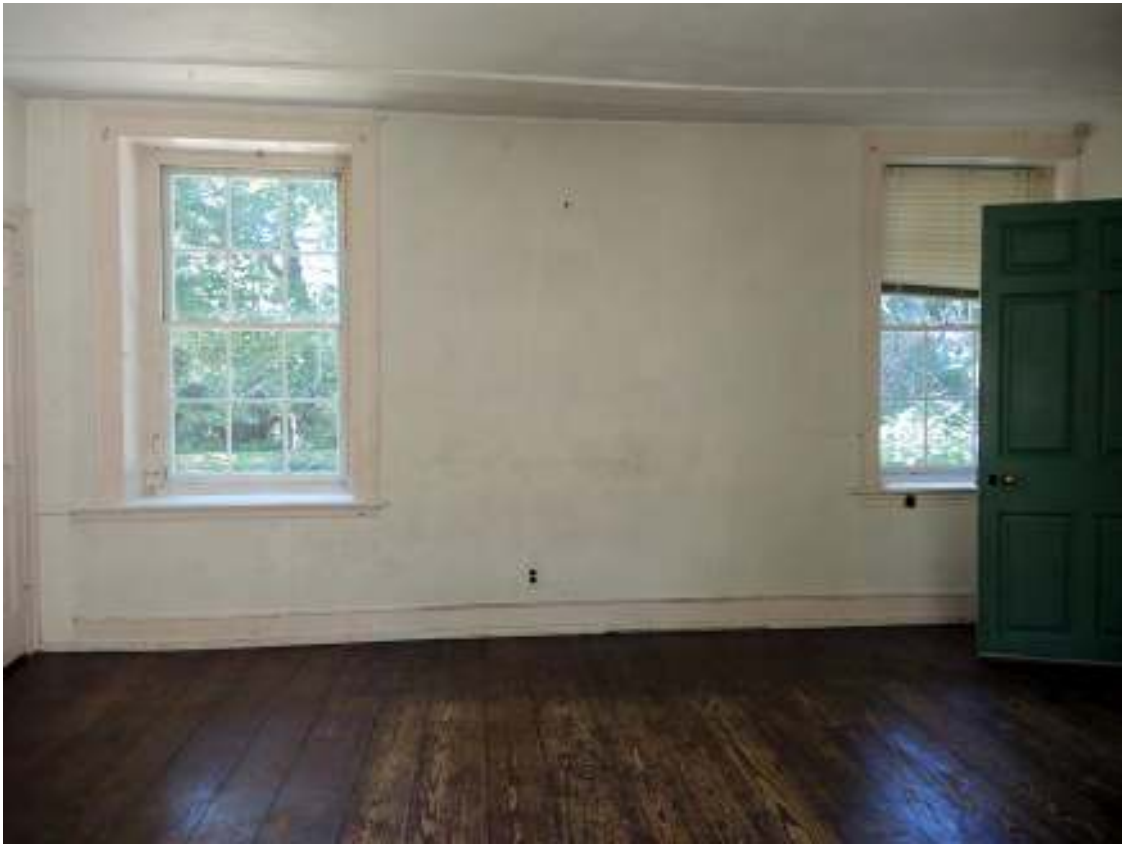
PHOTO 091 - Ell Interior, Room 107, West Wall; Framing Member Potentially Out of Plumb (09-14-2016, NTHP)
