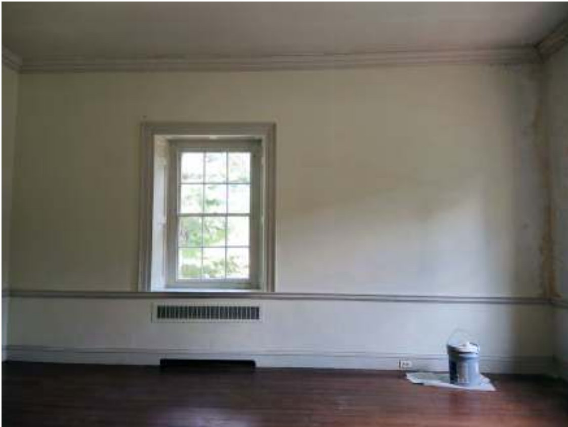
PHOTO 111 - Main Block Interior, Room 203, West Wall; Plaster Wall & Molding Damage at North Wall & Corner (09-13-2016, NTHP)
