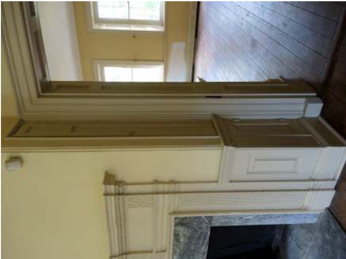
PHOTO 066 - Main Block Interior, Room 101, Detail of West Cabinet; Cracked Plaster and Paint along side of Fireplace Mantel (09-13-2016,...
