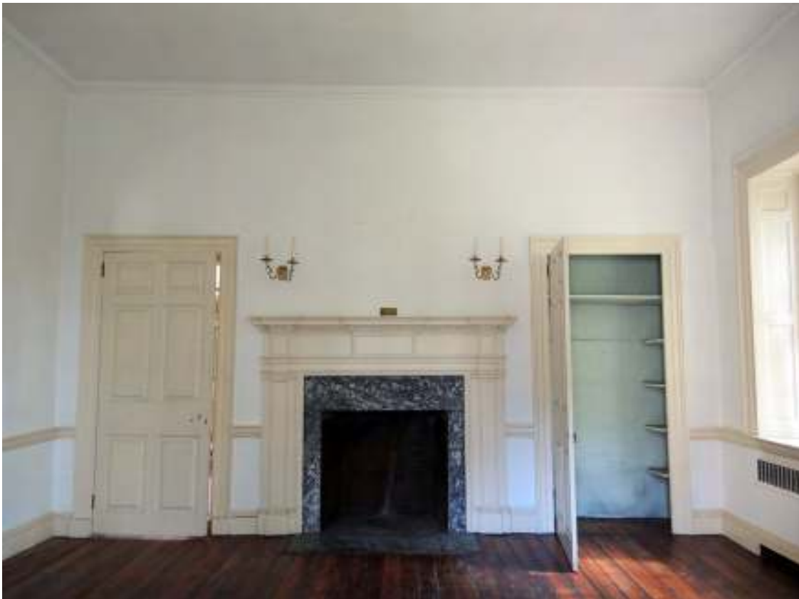
PHOTO 120 - Main Block Interior, Room 204, North Wall; Cracked Plaster from Ceiling to Wall above East Door (09-13-2016, NTHP)
