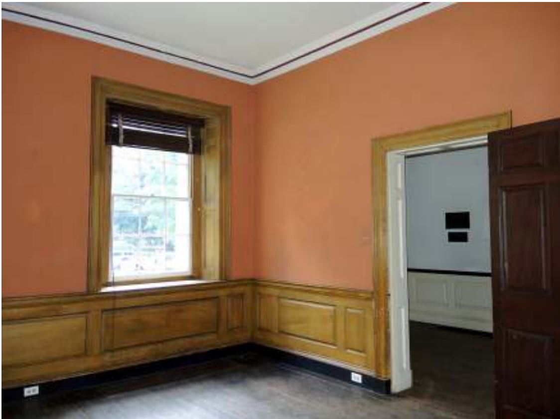
PHOTO 070 - Main Block Interior, Room 103, Northeast Corner; Uneven Wood Floor at East Wall, Window Sill Damage, Cracked Plaster in ...
