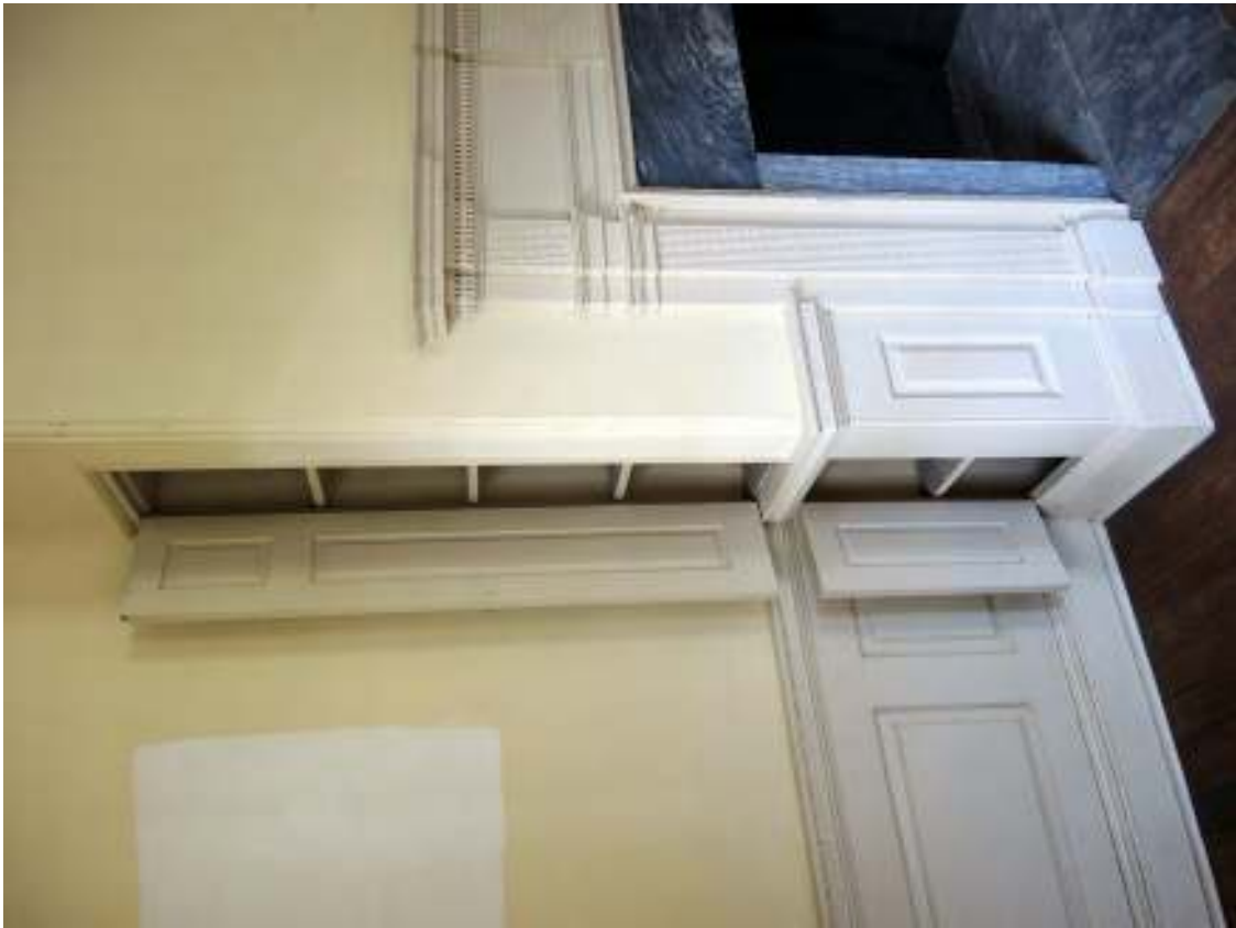
PHOTO 065 - Main Block Interior, Room 101, Detail of East Cabinet; Cracked Paint along side of Fireplace Mantel (09-13-2016, NTHP)
