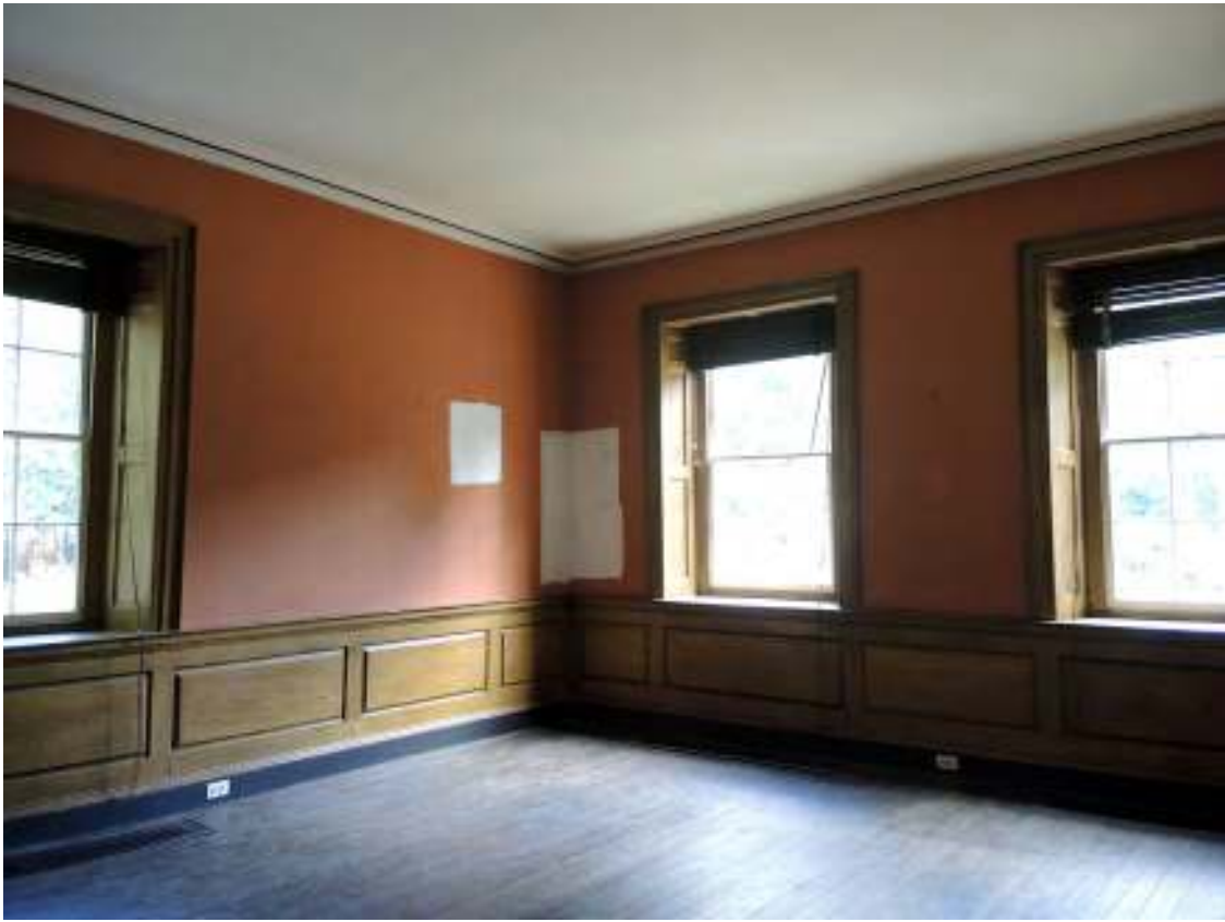
PHOTO 069 - Main Block Interior, Room 103, Northwest Corner; Uneven Floor at West Wall, Cracked Plaster Molding, Window Sill Damage...
