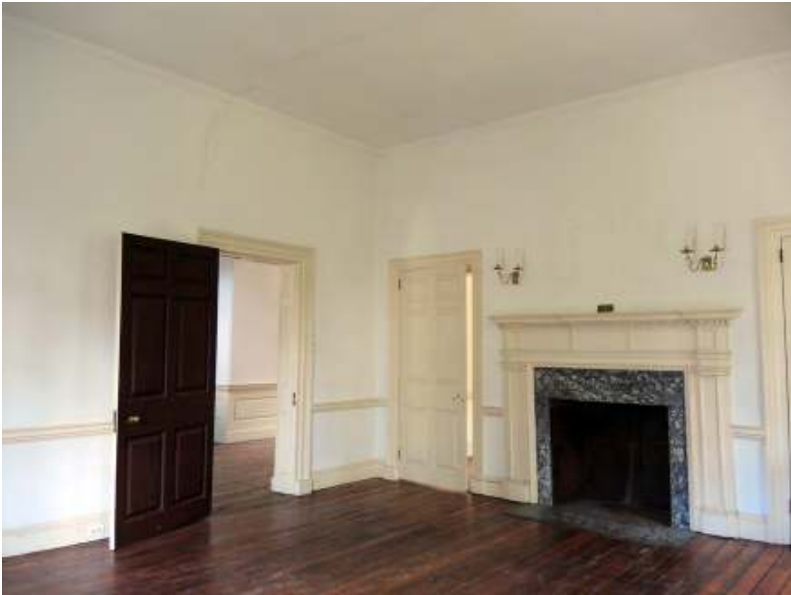
PHOTO 119 - Main Block Interior, Room 204, Northwest Corner; Cracked Plaster from Top of West Door to Across the Center of the Ceiling ...
