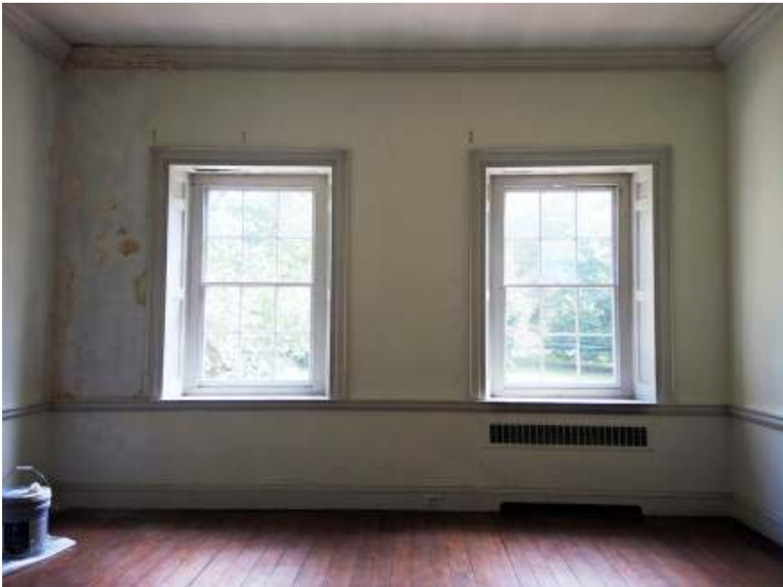
PHOTO 112 - Main Block Interior, Room 203, North Wall; Plaster Wall & Molding Damage at West Corner, Damaged Window Casings (09-1...
