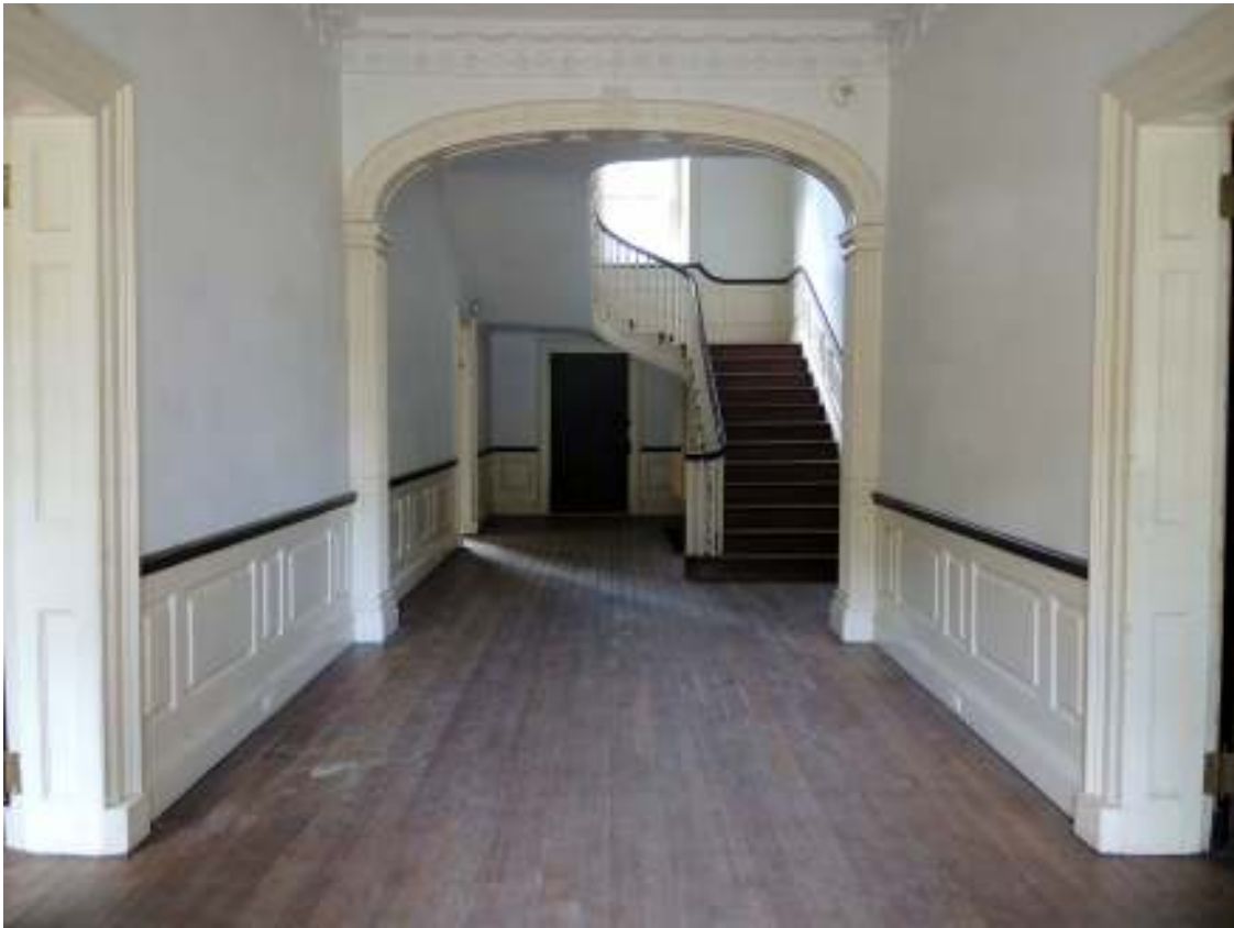
PHOTO 047 - Main Block Interior, Room 102, Looking Southwest; Wooden Arch Slight Separation from Wall (09-13-2016, NTHP)
