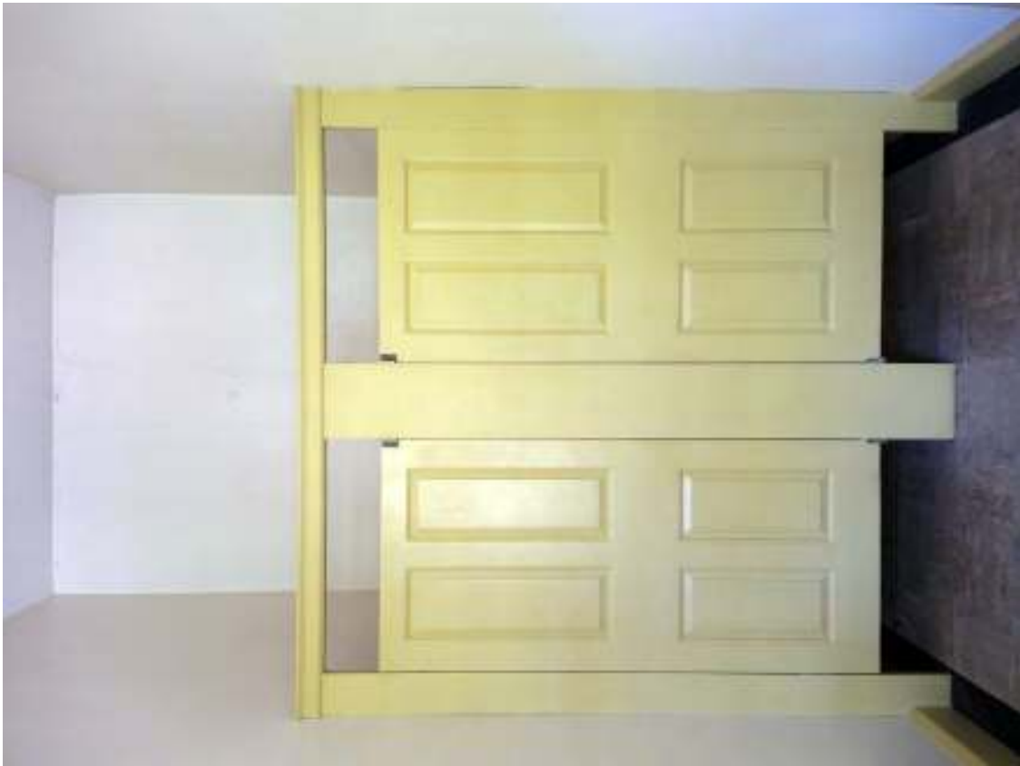
PHOTO 130 - Main Block Interior, Room 205A, East Wall; Two Cracks from Top of Wall Down, Plaster Depression at Top of Wall (09-14-20...
