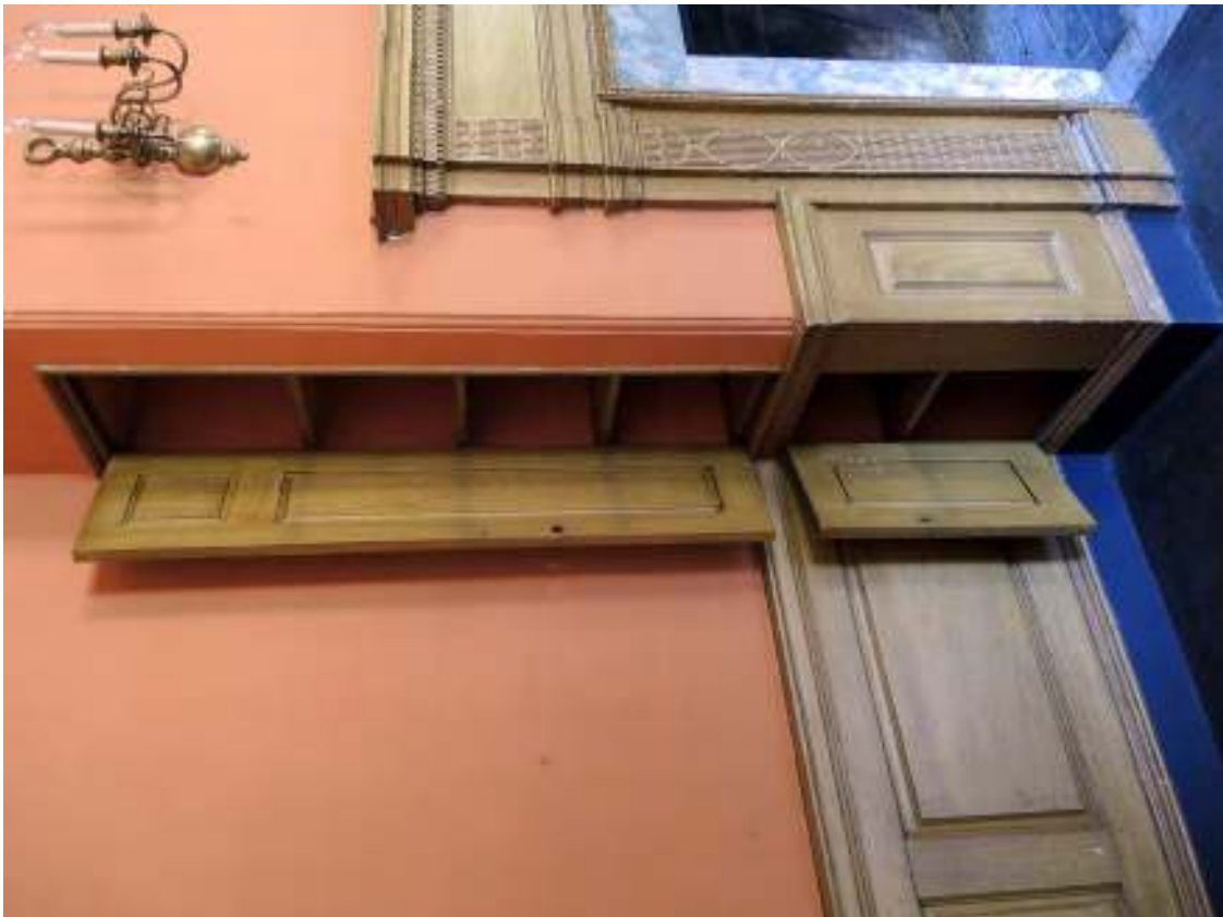
PHOTO 072 - Main Block Interior, Room 103, Detail of East Cabinet; Cabinet Hardware Missing (09-13-2016, NTHP)
