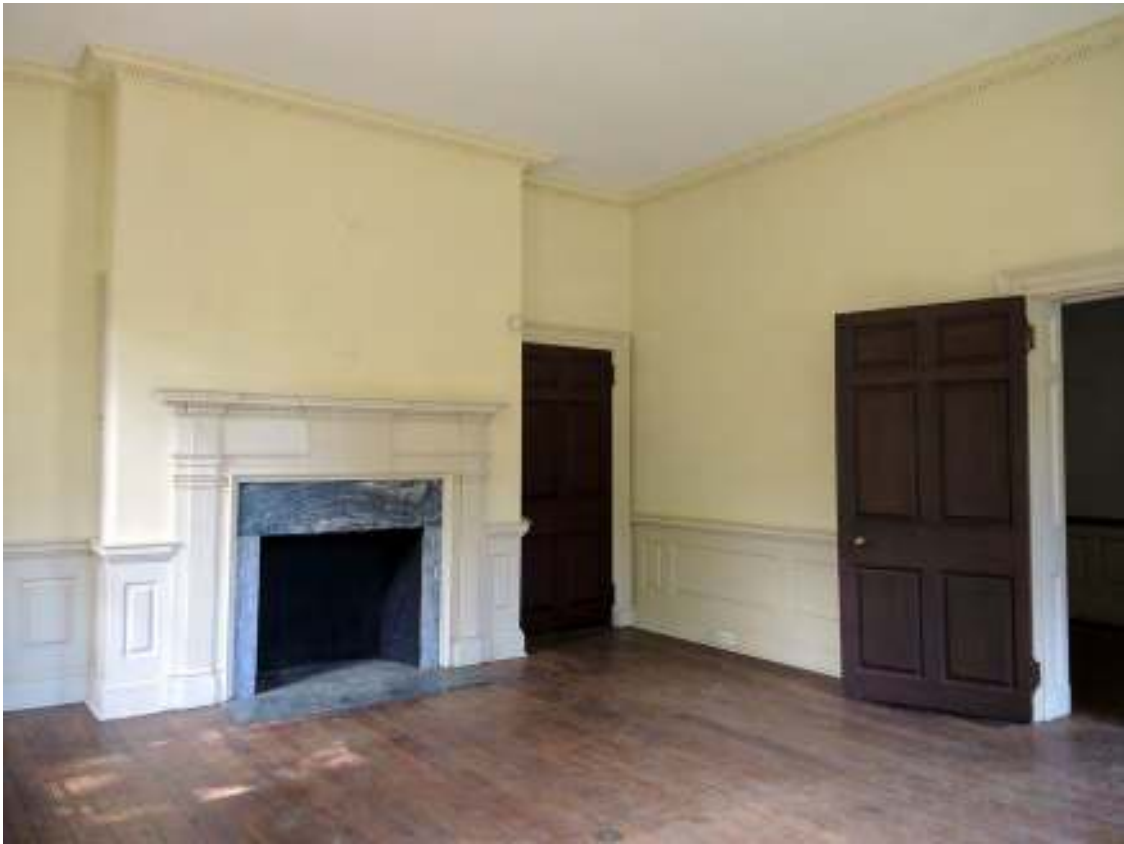
PHOTO 061 - Main Block Interior, Room 101, Southwest Corner; Cracks in Stone Fireplace Surround (09-13-2016, NTHP)
