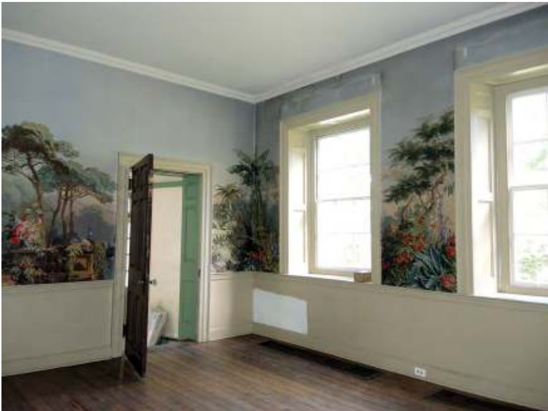
PHOTO 080 - Main Block Interior, Room 105, Southwest Corner; Plaster Molding & Ceiling Damage at Corner, Plaster Crack in West Ceiling...
