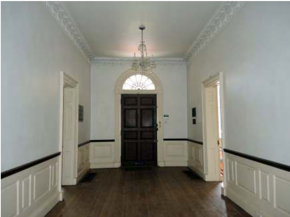
PHOTO 054 - Main Block Interior, Room 102, Looking Northeast; Plaster Crack in East Corner (09-13-2016, NTHP)
