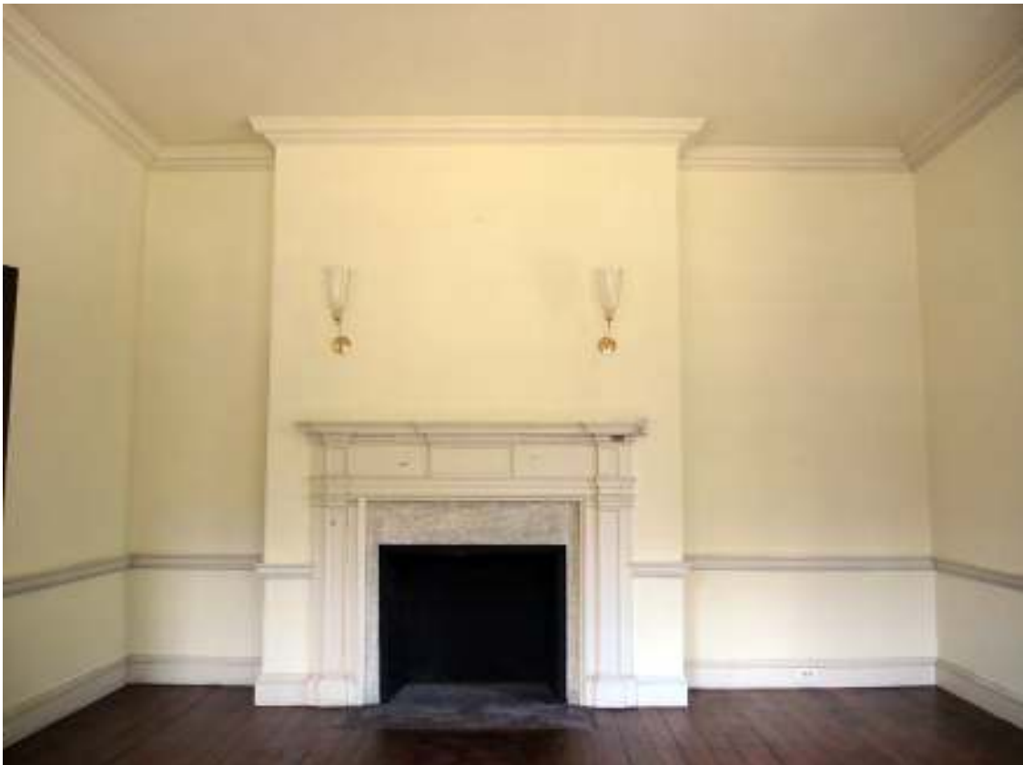
PHOTO 110 - Main Block Interior, Room 203, South Wall; Fireplace Mantel Missing Dentils (09-13-2016, NTHP)
