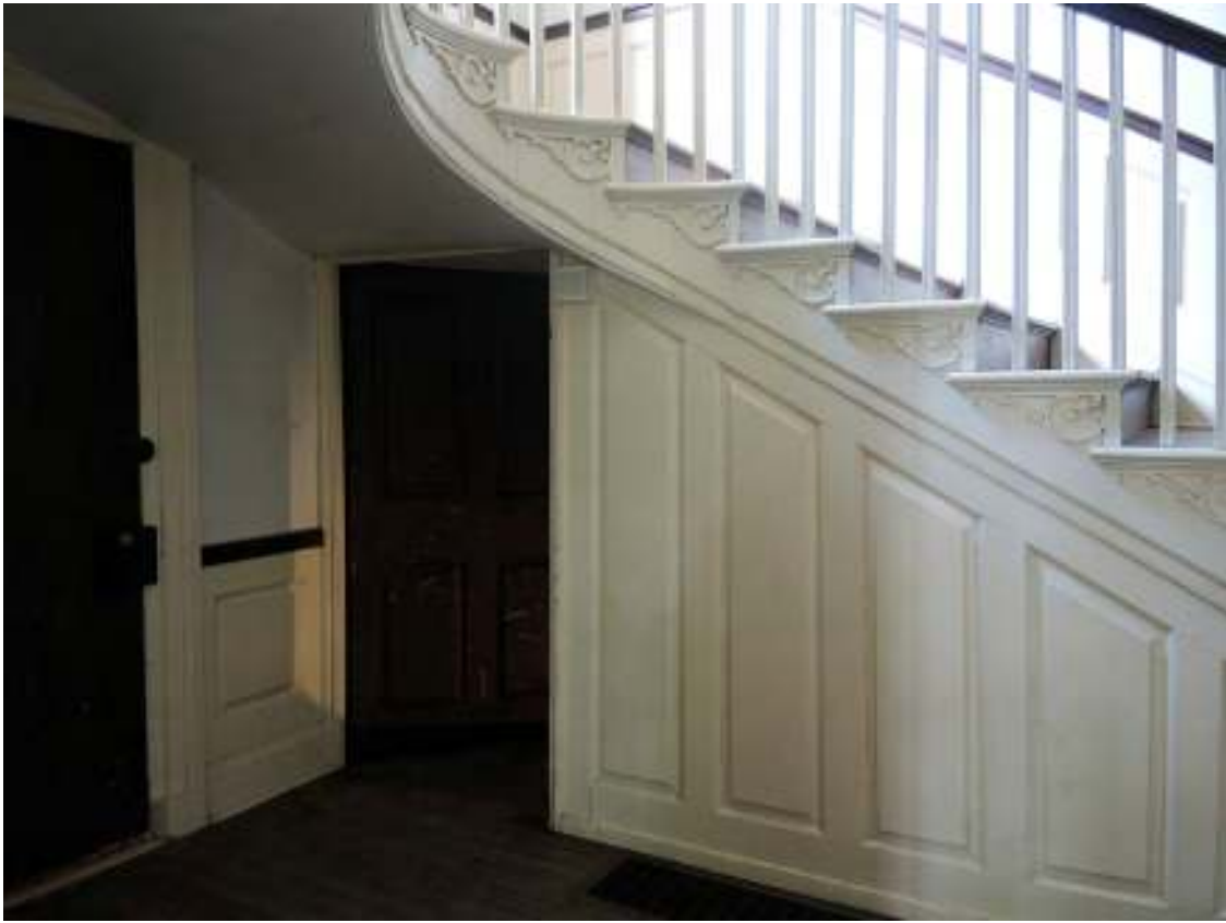
PHOTO 049 - Main Block Interior, Room 102, Looking West at Cellar Door; Cracks along Curved Stair Stringers (09-13-2016, NTHP)
