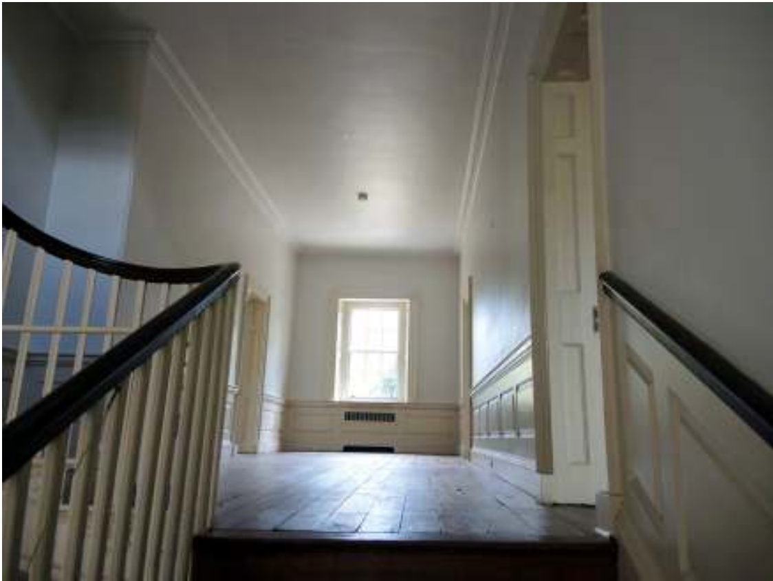
PHOTO 103 - Main Block Interior, Room 202, Looking Northeast; Holes in Flooring along East Wall (09-13-2016, NTHP)
