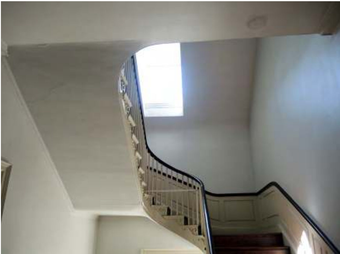
PHOTO 155 - Main Block Interior, Room 202, Looking Southwest; Plaster Damage on West Ceiling, Cracked Plaster Underside of Staircase...
