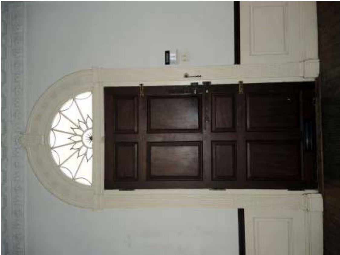
PHOTO 055 - Main Block Interior, Room 102, Detail of Entry Door; Cracked Plaster above Fanlight Keystone (09-14-2016, NTHP)
