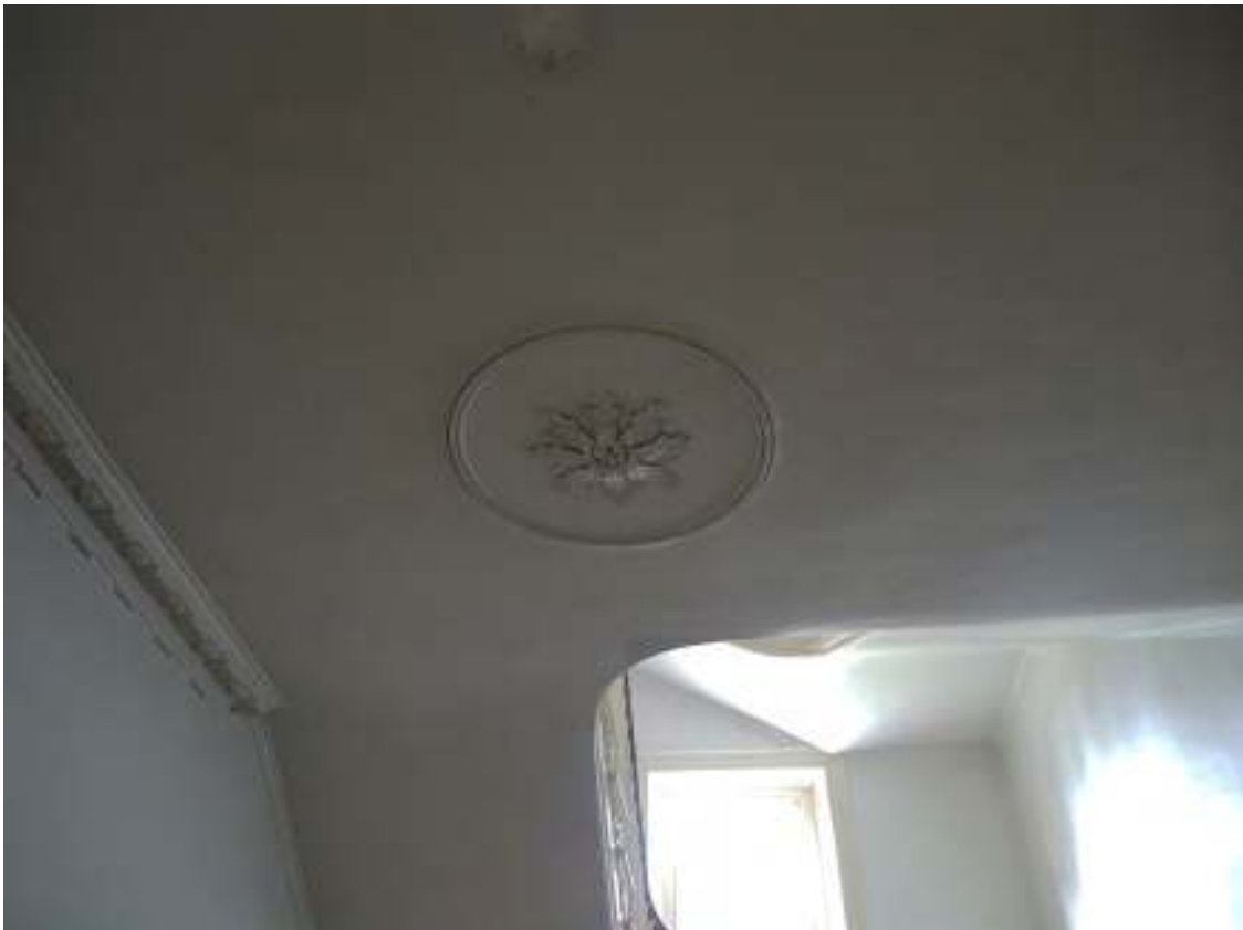
PHOTO 058 - Main Block Interior, Room 102, Detail of Plaster Medallion; Plaster Ceiling Discoloration Northeast of Ceiling Medallion (09-13...
